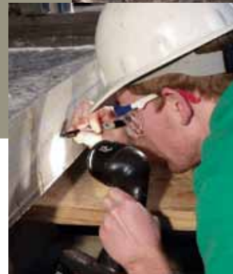
Nicholas Mascitelli CE '12 maps cracks in a reinforced concrete beam.
