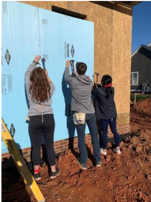
7 - Working together to put up Styrofoam insulation on a house in Hickory
