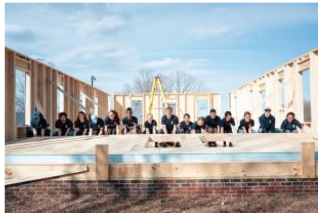
5 - My group putting up the fourth wall for the house we were building in Hickory, North Carolina
