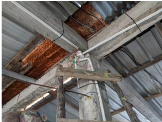
29 - Electrical wiring system connected to the lightbulbs
