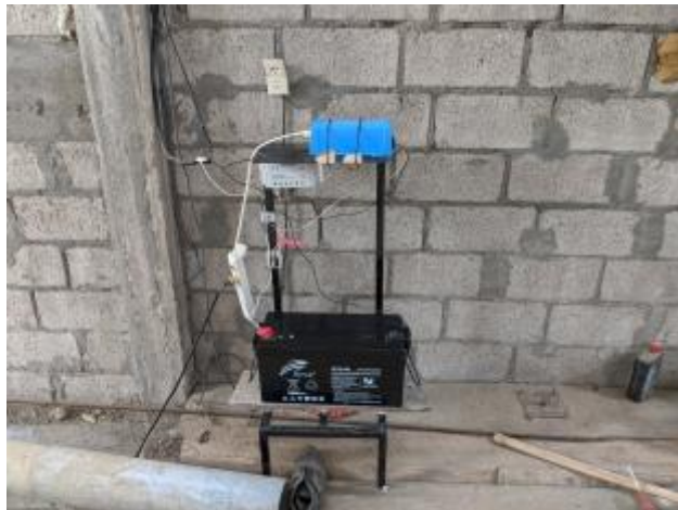
27 - The battery system installed and wired to the solar panel to power a house
