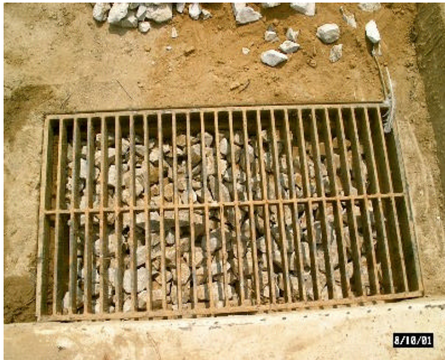
A5: Storm sewer inlet on north end of traffic island is filled. The grate is later paved over, diverting flow into the traffic island.
