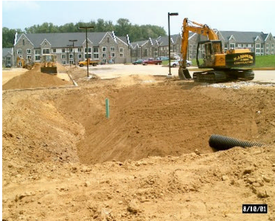
A7: Monitoring well is placed within infiltration bed.
