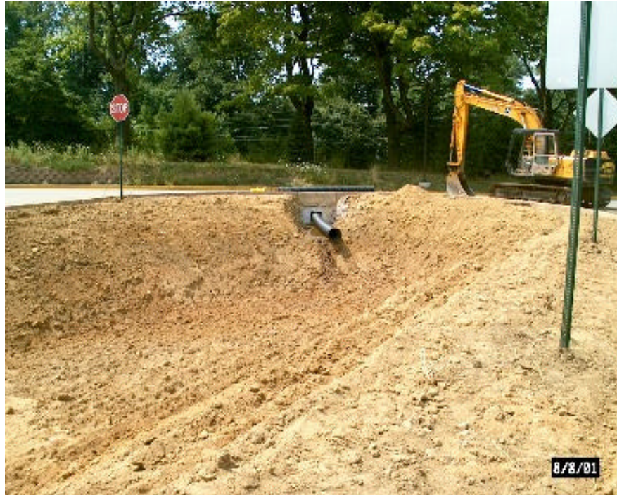
A3: Storm sewer inlet is blocked, and inlet pipe is added.
